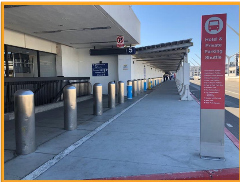
Departures Level temporary pedestrian sidewalk extension and canopy to be demolished starting this week
