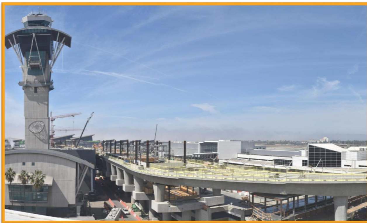
As captured from a construction camera atop the Theme Building, this view shows the APM guideway and CTA Center Station over Parking Structure 2A and, in the distance, Parking Structure 2B
