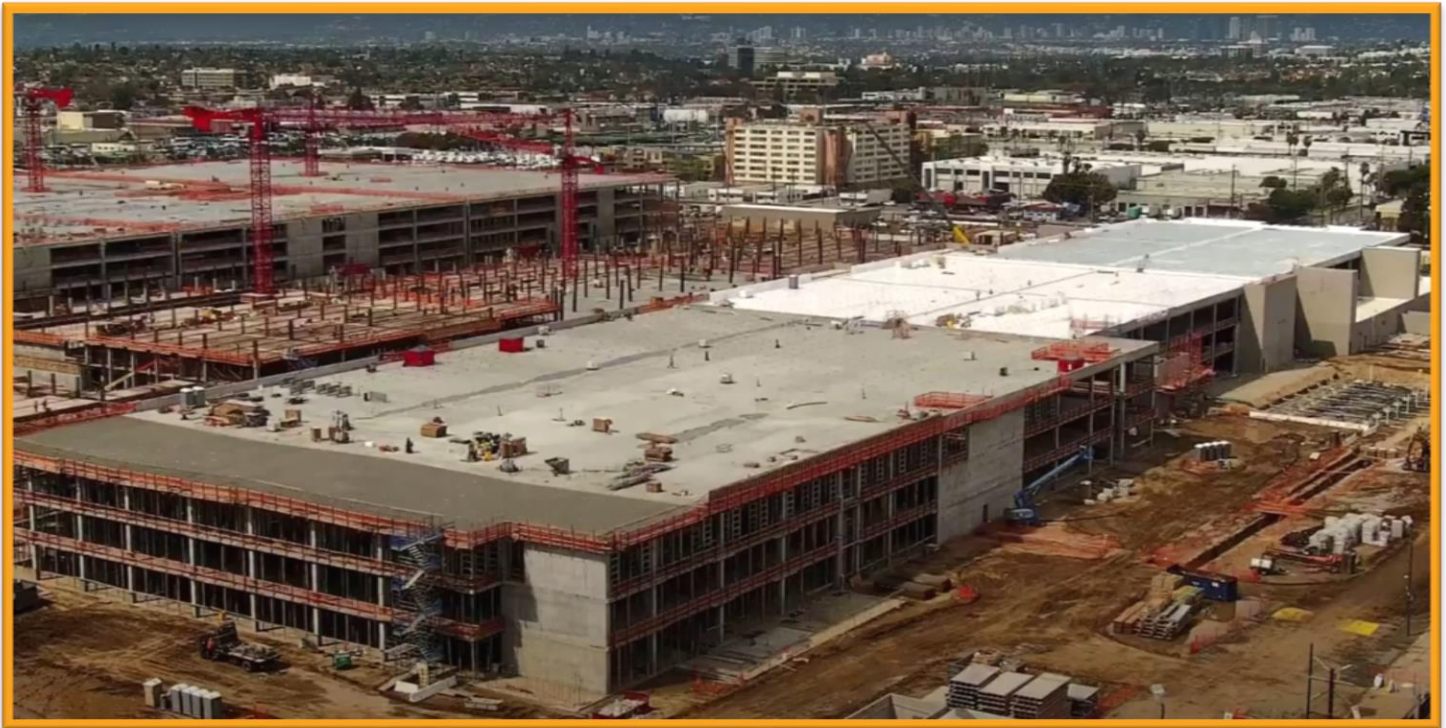
ConRAC final rendering (top) and current construction progress (bottom) following the final concrete pour for the Quick Turn Around building
