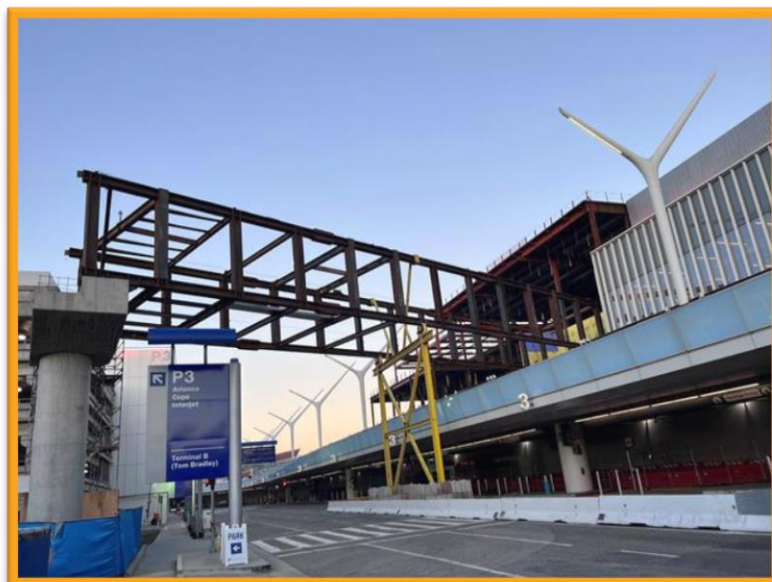
The Terminal 3 Pedestrian Bridge is the third out of six CTA Pedestrian Bridges to be installed
