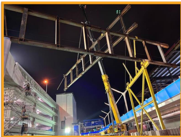
A 97,000 pound steel truss is lifted into place at Terminal 3 with the help of a 350-ton crane
