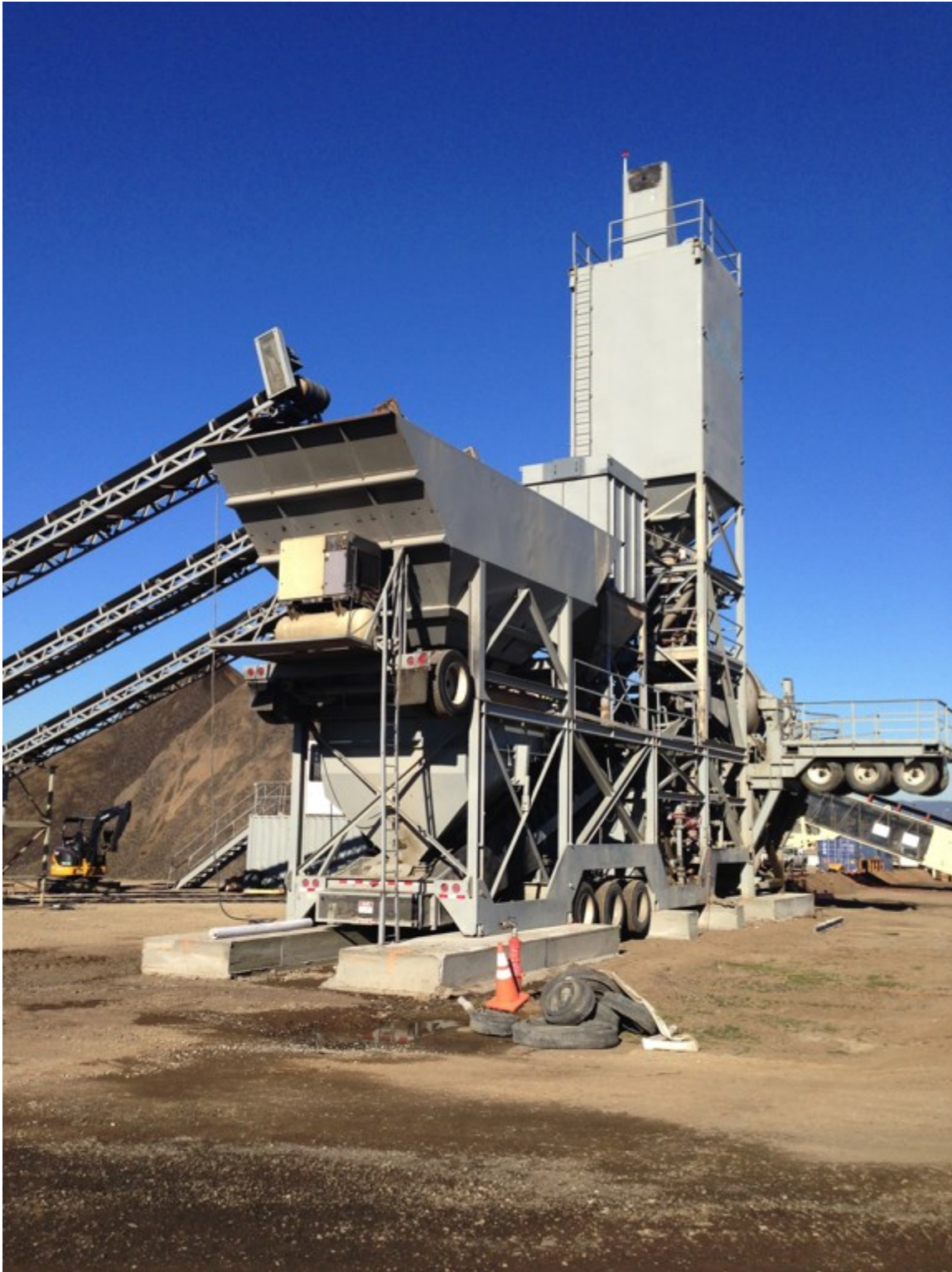
Figure 3.3-3: Concrete Batch Plant Undergoing Final Assembly in Preparation for Taxilane T Construction
