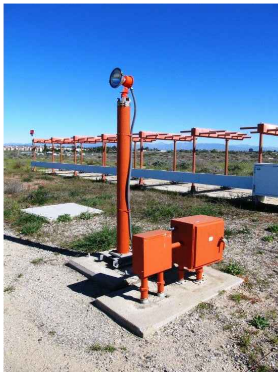
2. View of single-pole flashing station facing northeast. 1/
