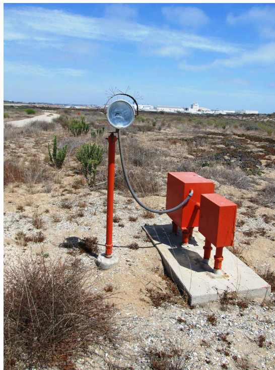
2. View of flashing Station facing east.
