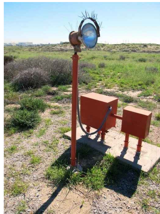
3. View of single-pole flashing station facing southeast.
